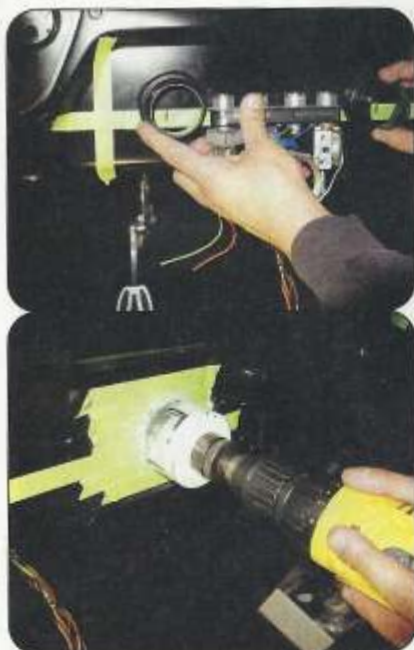
The spot where the holes are to be cut for the vents and the controls are measured out and cut.
