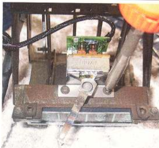
Then you'll attach the new fan blower switch to the top of the control panel.
