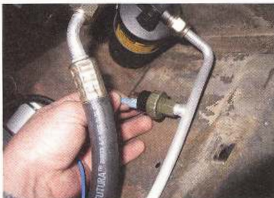
Attach the wire from the control panel to the binary switch. From the binary switch, run a wire to the A/C compressor.
